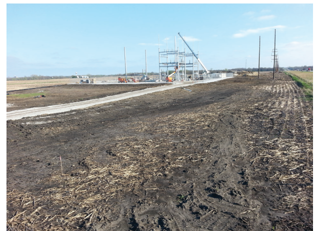
CIPCO has deployed Sensera Systems' MC-68 Model solar/wireless site camera — featuring 100% solar operation 24/7, time-lapse, live video streaming, built-in DVR, and LiveView — on the electrical substation project.
